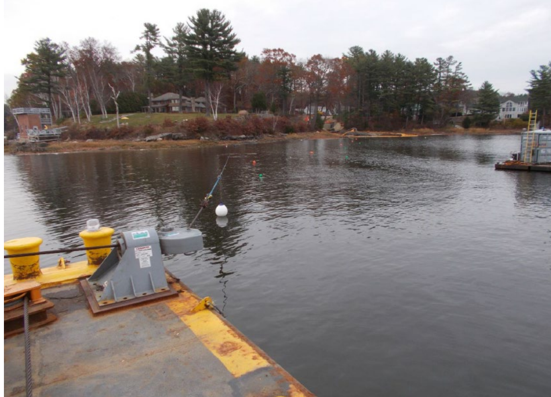
Cable 3 installation approaching the eastern landfall (Gundalow Landing). Port bow anchor wire in view and diver barge on the right side of the frame. Photo courtesy of Durocher Marine.
